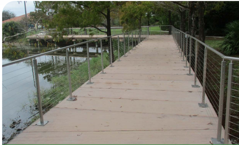
Sabal Pines Wood Boardwalk Replacement
